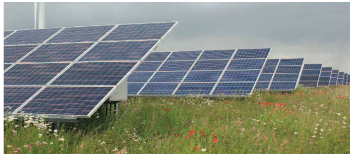
Figure 30, PV Farm A section of 5MW ground mounted PV systems at Westmill. (Picture: TV Energy)
