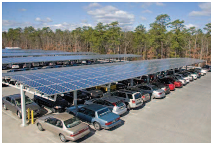
Figure 31, Solar PV array over parking area The Richard Stockton College of New Jersey parking array
